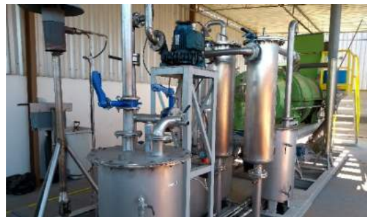
Figura 12 – Side view of the filtration system
